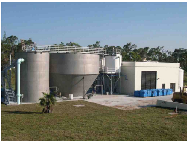
Figure 1: R.L. Platt WTP (4 MGD) at the Village of Palm Springs, Florida.
