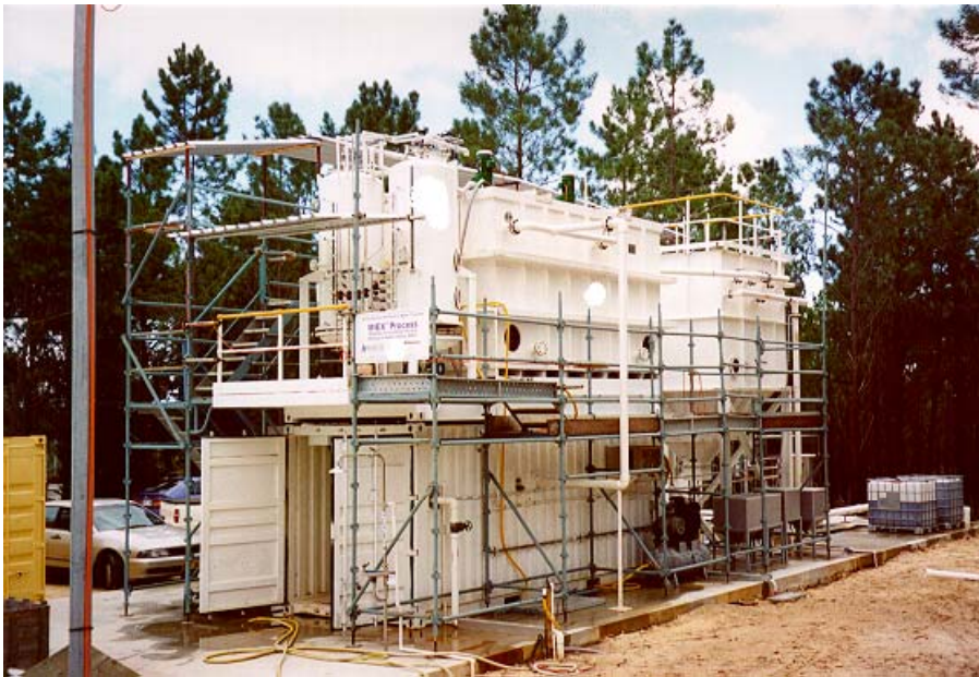
Figure 3: 0.26 MGD (1 MLD) MIEX ® Resin Pilot Plant at Wanneroo, WA, Australia
