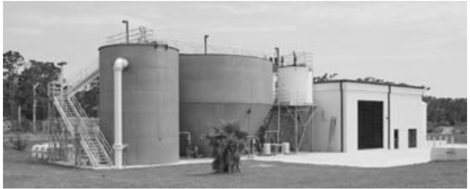
Palm Springs, FL, is the first to use the Orica MIEX® DOC technology in the U.S. Pictured are the contactor tank (foreground), resin recovery settler (center) one of the two batch resin regeneration tanks (white elevated tank) and the resin handling building.
