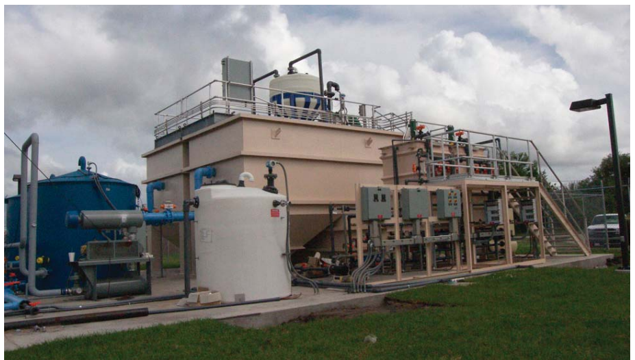
Figure 3: 1.4 MGD MIEX® Treatment System at Wedgefield, FL
