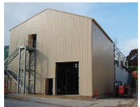
Figure 1: 60 MLD MIEX ® System at Yorkshire Water's Albert WTP, the first of three MIEX ® Plants to be installed by 2010
