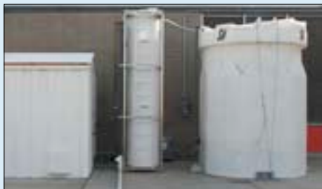
Photo: 50 gpm MAGNAPAK® System at the DWR San Luis Field Division WTP
