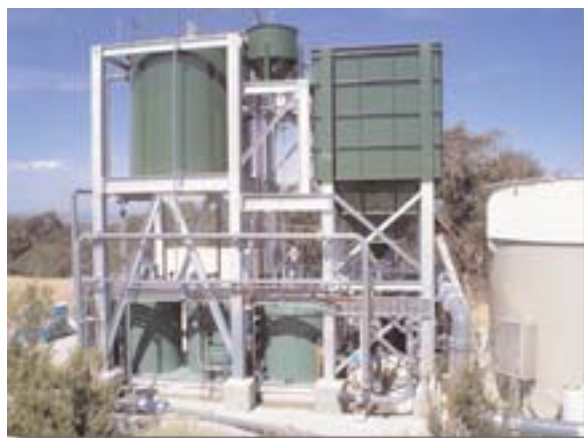
Airey's Inlet 280 gpm MIEX ® installation.
