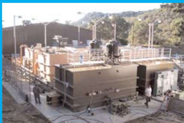
1 MGD MIEX ® System in foreground.
