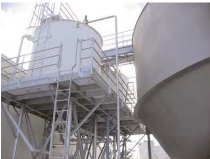
RL Pratt WTP Resin Regeneration Tanks
