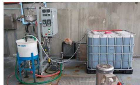
Figure 8: NF Unit Treating Waste from a full-scale MIEX® System in Florida
