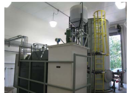
Figure 1: MIEX ® System at the Newport, Maine Water Treatment Plant
