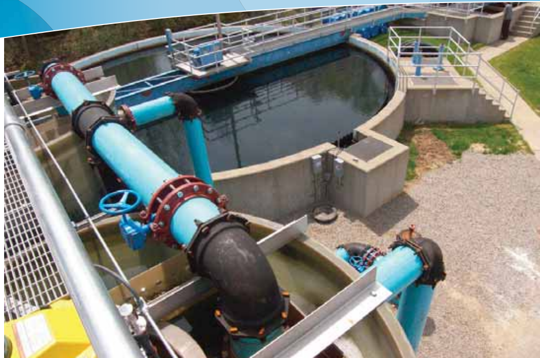
Figure 4: Raw water is first treated by the MIEX ® Process (front left) then flows to downstream coagulation and clarification (rear).
