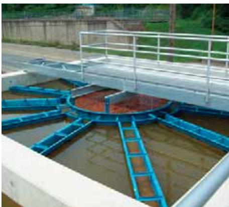
Figure 1: Settling vessel at Portsmouth, Ohio MIEX ® Installation
