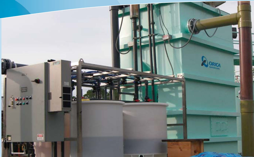
Figure 2: 250 gpm MagnaPak® System at Cedar Key WTP
