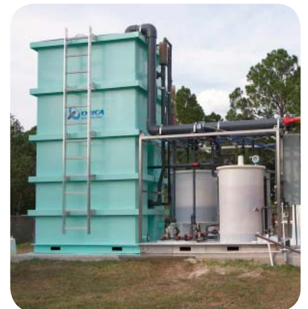
Figure 1: MIEX ® System at Cedar Key Water Treatment Plant
