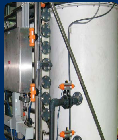
Regeneration System at the Ocean Shores, WA WTP
