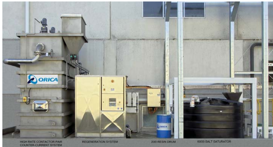
Figure 1: MIEX® System at Visy Industries
