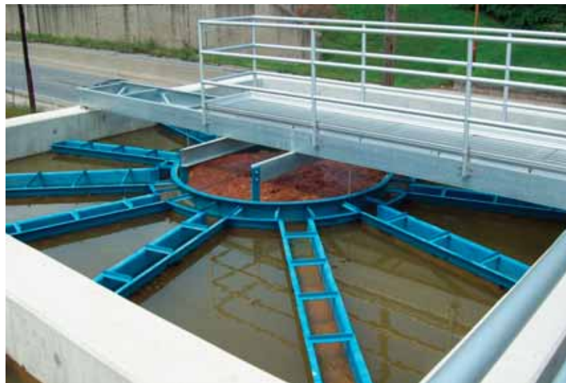
Figure 1: Settling vessel at Portsmouth, Ohio MIEX® Installation
