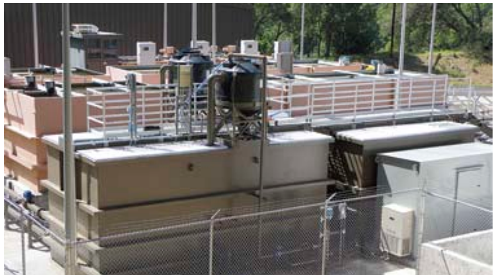
Figure 1: MIEX® Installation (foreground) at the Green Valley WTP
