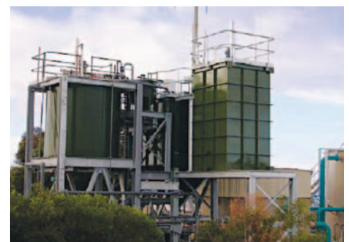
Figure 1 MIEX ® High Rate Contactor (foreground) with Dual Stage System (background)
